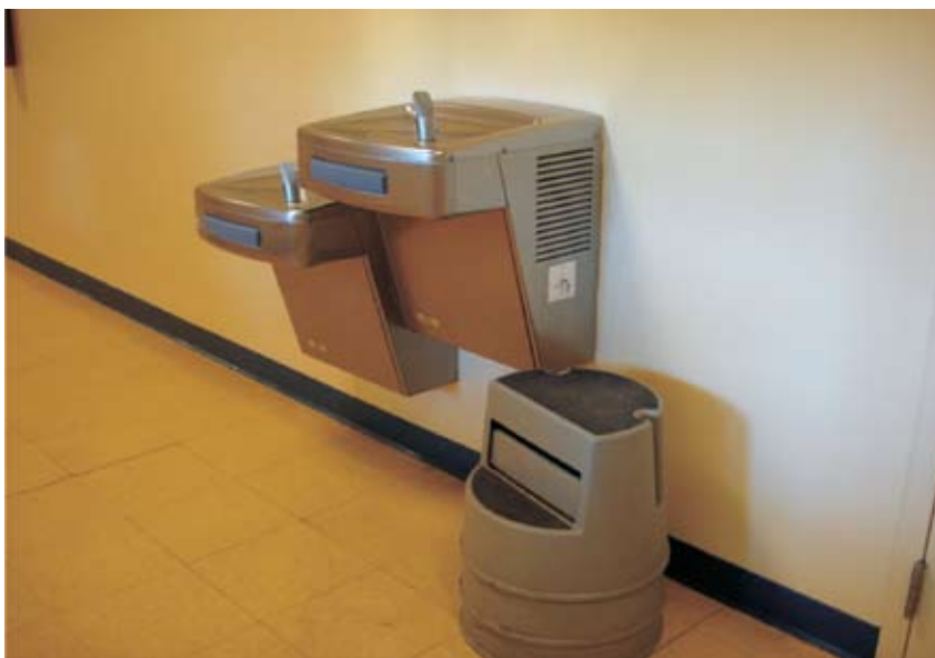
Fig 8: Drinking water facilities to accommodate different heights and helpful for children on wheelchair
